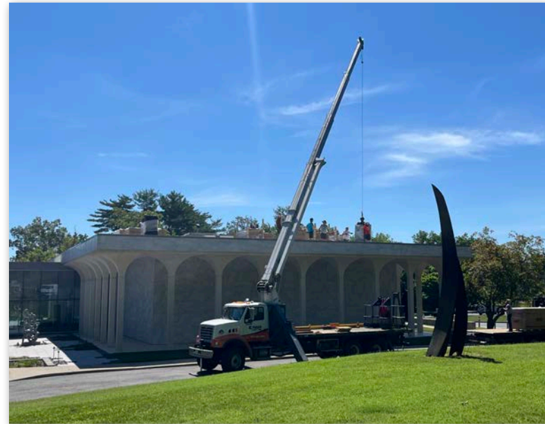
The cranes arrived in June 2024 to lift solar panels onto the roof of the original Mitchell Museum building. The new system includes 283 panels and should generate roughly 40% of the museum's energy usage.
